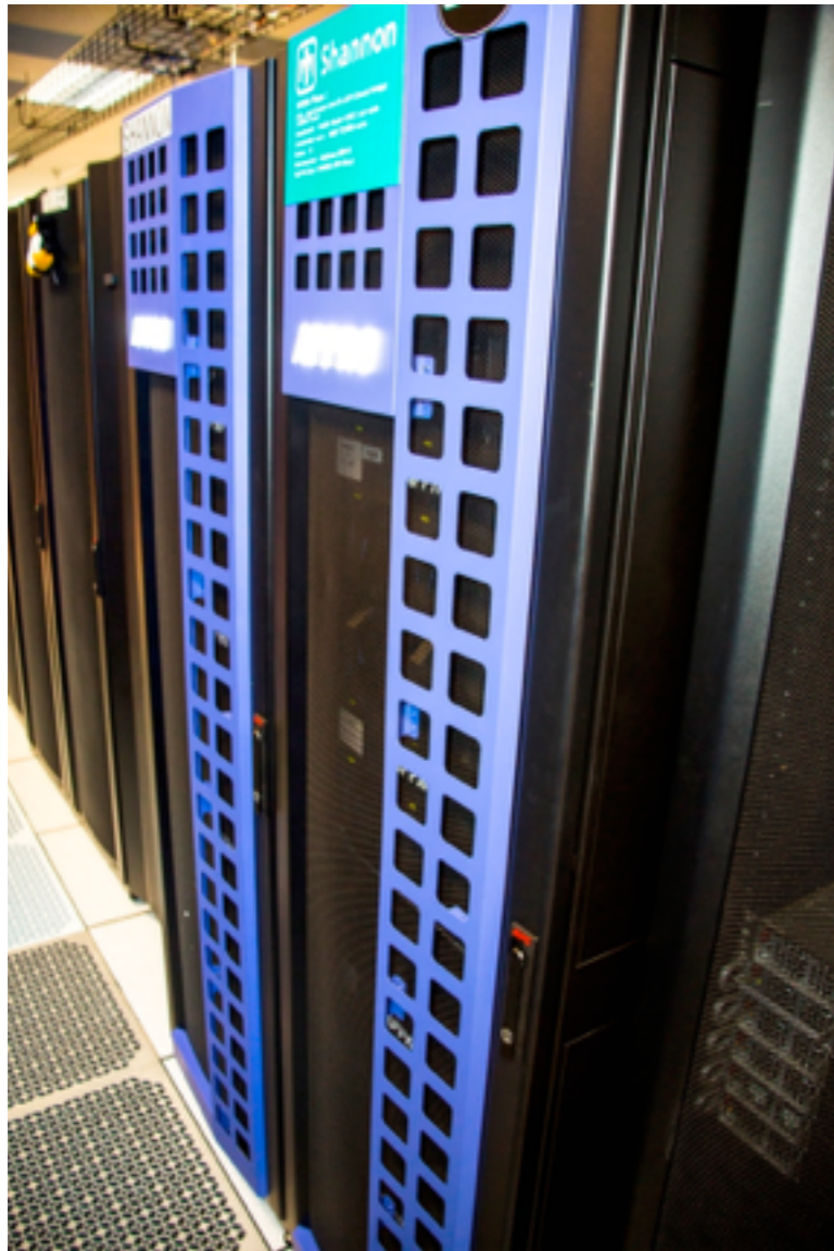
Shannon testbed at Sandia National Labs
